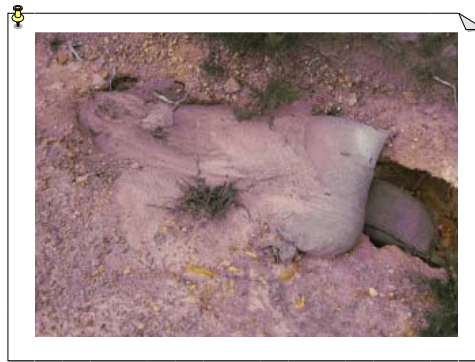
“hard working sand bag” : A couple of sand bags in an eroding road drain—one rain event and it filled to the top with sediment! Submitted by Matthew Hulse, Braidwood
